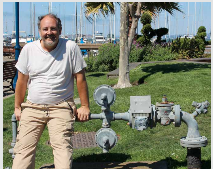
The “flange academy” is twice as fun in open-air installations – discovered by M. Döller in San Francisco.
